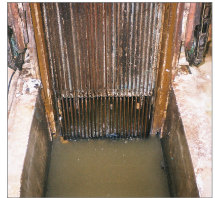
ABOVE: Rusted Bar Screen
